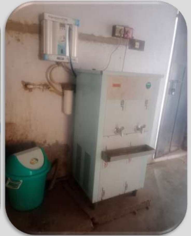
Sanitation and Drinking Water
